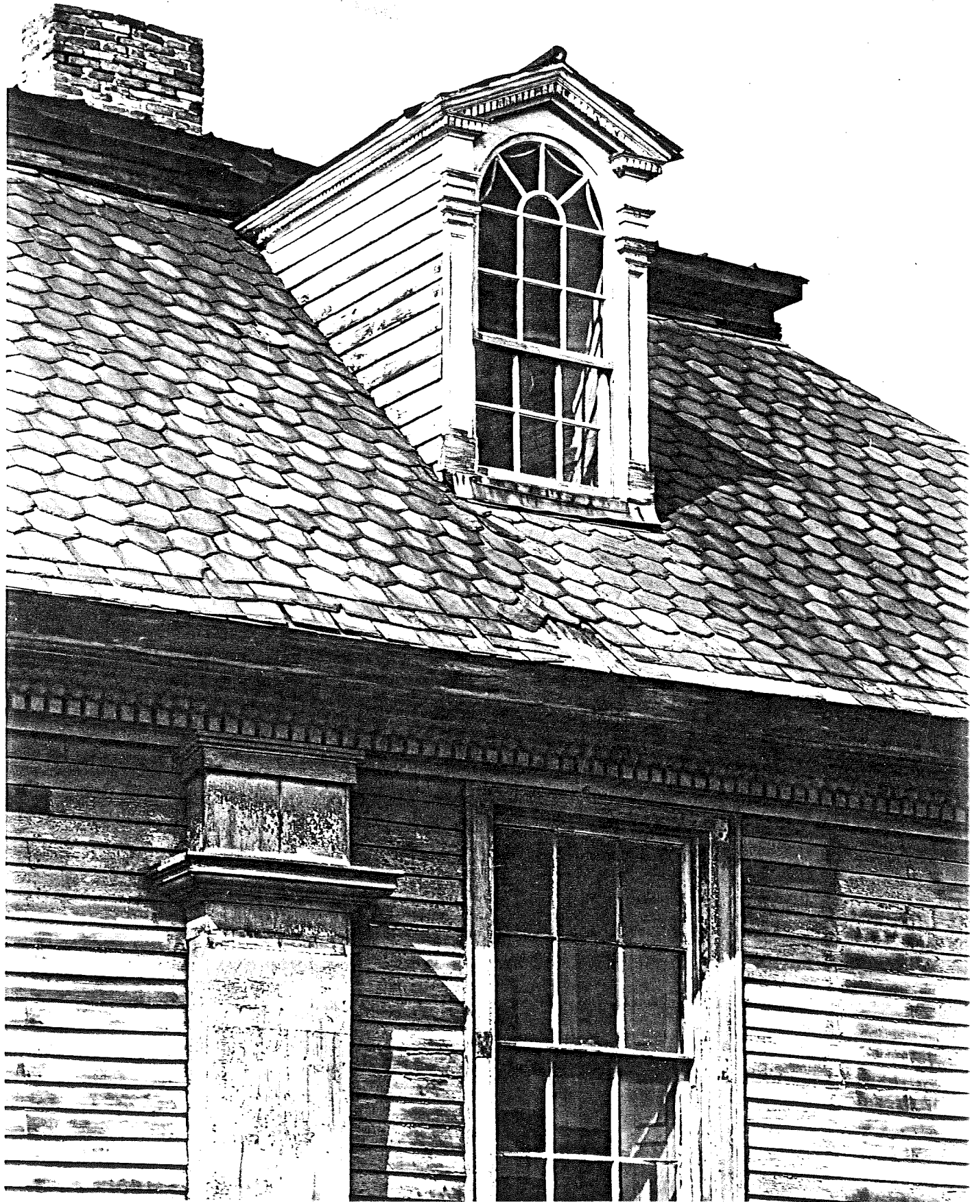
Fig. C-9. Shirley-Eustis House, east dormer, cornice, and pilaster capital detail showing seam at removed neck molding, possible evidence of former entablature. Arthur Haskell photo, 2 September 1939. (SPNEA Neg. 13204 AH)
